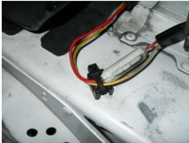
Use a zip-tie to reattach the wire at the bottom of the tank.
